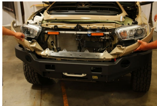
Step 9: Now remove bumper *Customer's Tacoma has aftermarket bumper, you will have to loosen the 8 bolts located under the bumper*
